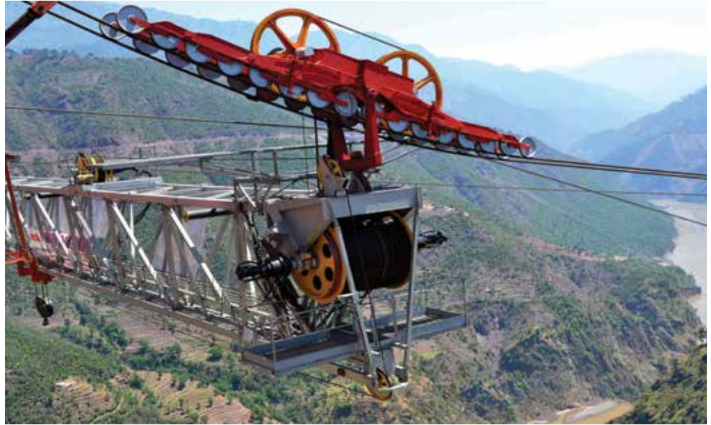
The cable crane at Chenab Railway Bridge Project can handle loads up to 34 tonne on single hook
