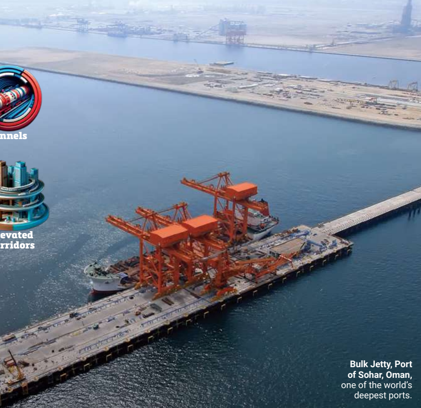
Tema to Mpakadan Railway Project, Ghana , the country's largest railway project, including the construction of the world's deepest raker piles in the Volta River
