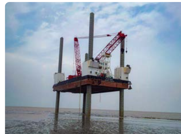
9 Large-capacity Jack ups (200–750 tonne)
